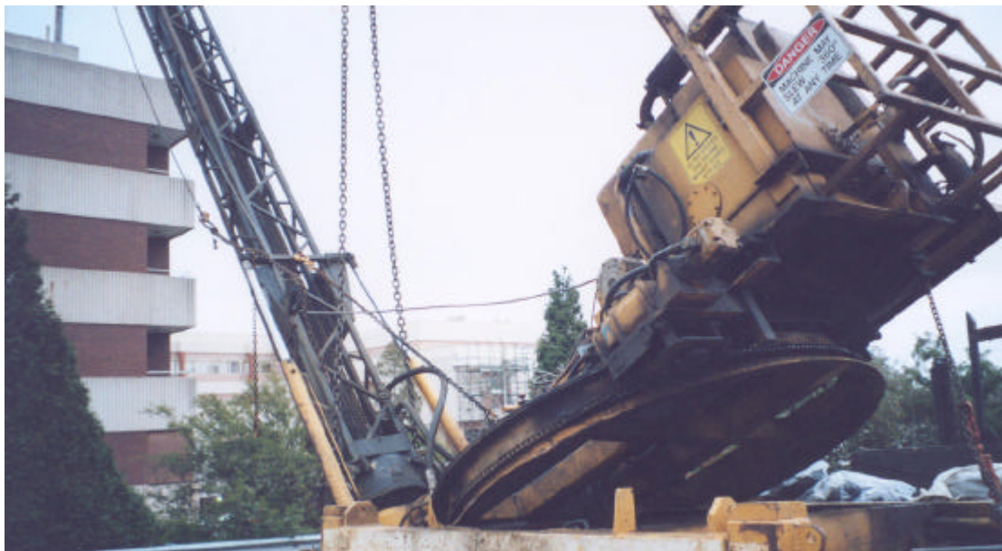
The damaged rig
