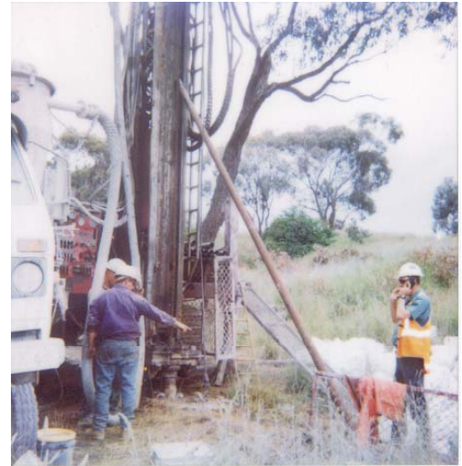
Figure 2. Drill rod leaning against rig mast, end 'speared' into metal mesh guard. Clamshell and main winch at top (7/8) position on rod.
